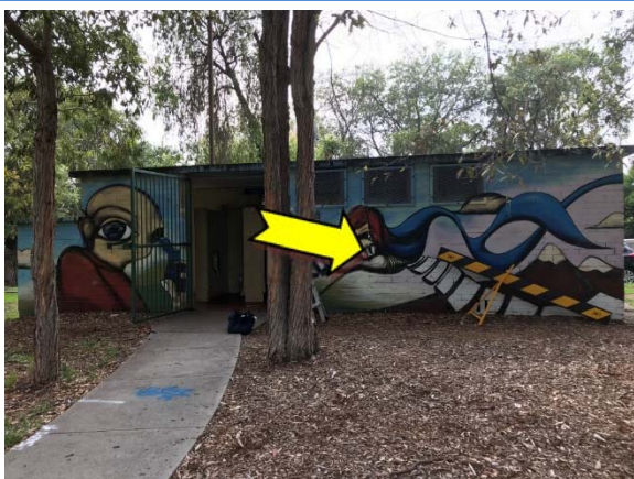
Photo 5. Exterior, throughout, walls, graffiti – suspected lead-containing various upper coloured paint systems.
