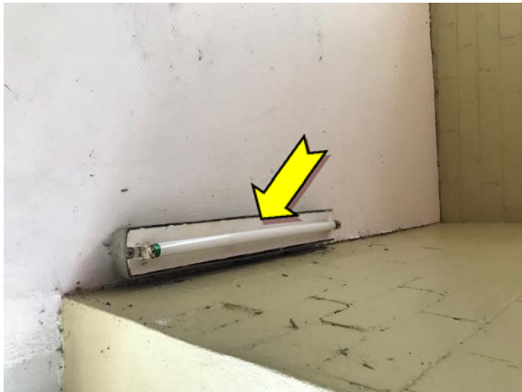
Photo 3. Interior, throughout, single tubed fluorescent light fittings – suspected PCB-containing capacitors.
