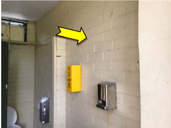
Photo 7. Interior, throughout, walls – suspected lead-containing light yellow upper paint systems.
