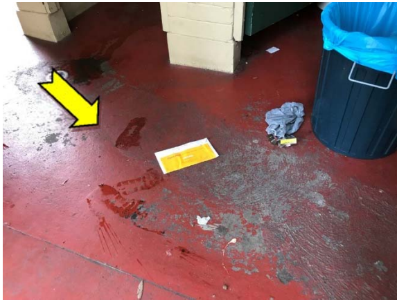
Photo 9. Interior, throughout, floor – suspected lead-containing red upper paint systems.
