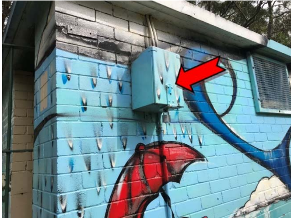
Photo 1. Exterior, south-east elevation, electrical backing board – suspected asbestos-containing bituminous backing board
