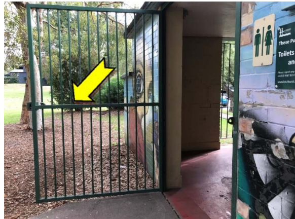
Photo 4. Exterior, throughout, door and frame – suspected lead-containing dark green upper paint systems.
