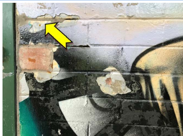
Photo 6. Exterior, throughout, walls – suspected lead-containing white and grey lower coloured paint systems.
