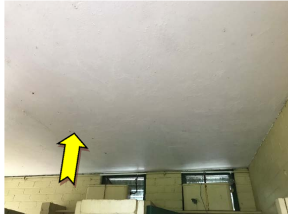
Photo 8. Interior, throughout, ceiling – suspected lead-containing white upper paint systems.
